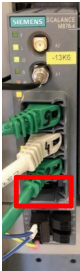
Figure 3-33 SCALANCE router with marked port for the ext. EMS
